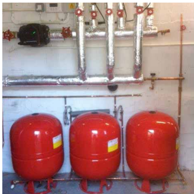
Old Building converted to a Plant Room
