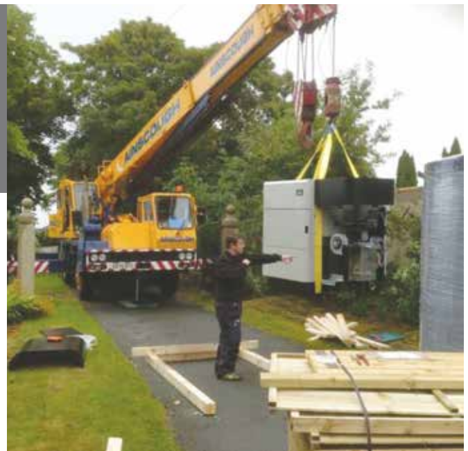
Ainscough Crane Hire lifting 199kW E-COMPACT in through roof of Plant Room
